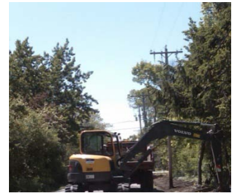
DCUS crews complete ditching project on Bay Point, Tennyson, and Regent Road
